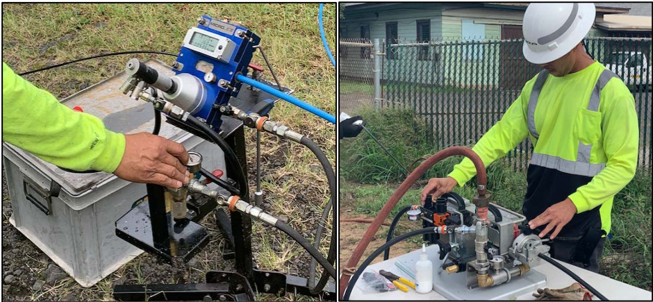
Figure 16 Cable Jetting Machines
