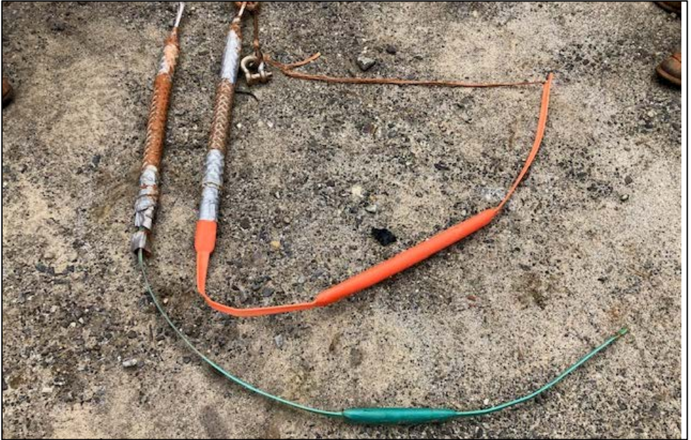
Figure 10 Tensile Failure of Conduit Due To Overstress During Pulling
